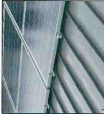
SOLAR PANELS ON ROOF 8
