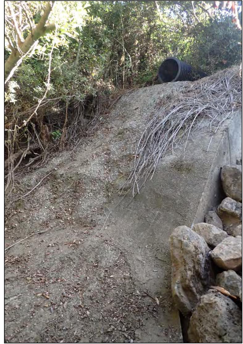
Photograph 3. View of the existing outfall and concrete from San Pedro Creek (taken 09/20/2019).
