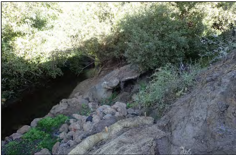
Photograph 2. View of the existing outfall and concrete from the north bank facing downstream (taken 09/20/2019).
