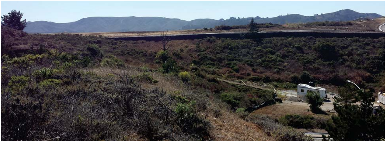
View 8: View from the project site looking south at the undeveloped hillside and roadway under construction for the new housing development across Fassler Avenue.
