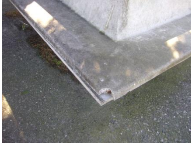
Chipped bench corner
